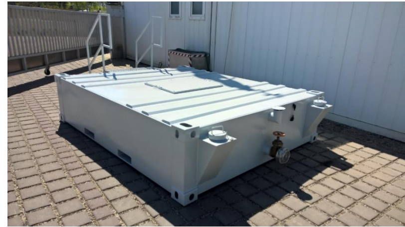
10 FT Septic-tank Mobile dry well
